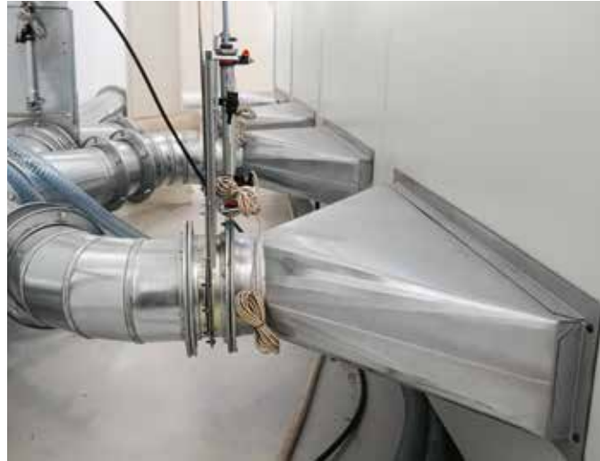
Dust extraction system for effective air recirculation and combating dust inside the work area
